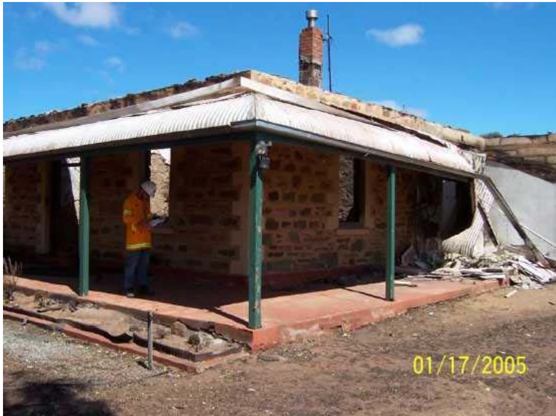
Surveying the damage to a house in Charlton Gully, near Port Lincoln.
