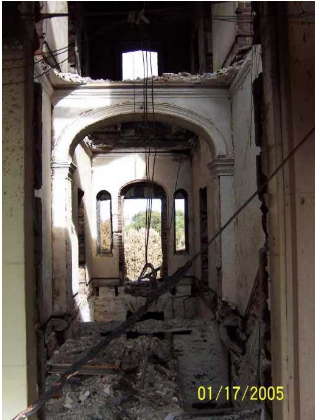
Interior of a destroyed heritage building in Green Patch, near Port Lincoln.
