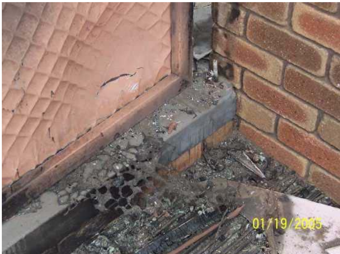
Close up of building damage in North Shields, near Port Lincoln.
