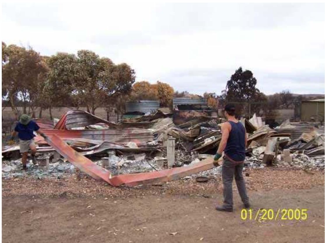
Cleaning up a building destroyed in Wanilla, near Port Lincoln.
