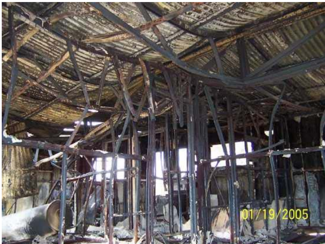
Interior of a building destroyed in Whites Flat, near Port Lincoln.
