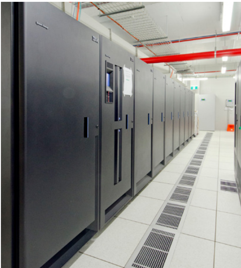
Figure 2. Data storage server racks. Information stewardship and delivery of high quality data to clients in the formats they require is an important role for Geoscience Australia.
