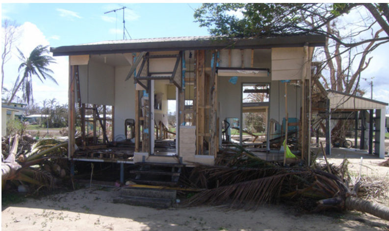
Figure 1. Storm surge damage due to cyclone Yasi, 2011.
