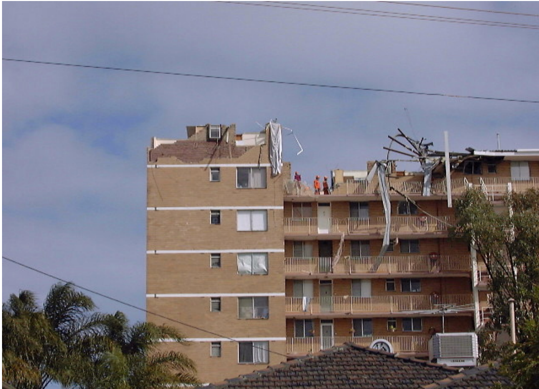
Plate 2.3: Damage to apartments in Fremantle, 25 August 1999 (Courtesy of BOM)
