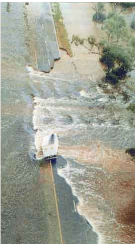
Flood damage to the Mitchell Highway near Nyngan, New South Wales, April 1990 Photo courtesy: Emergency Management Australia.
