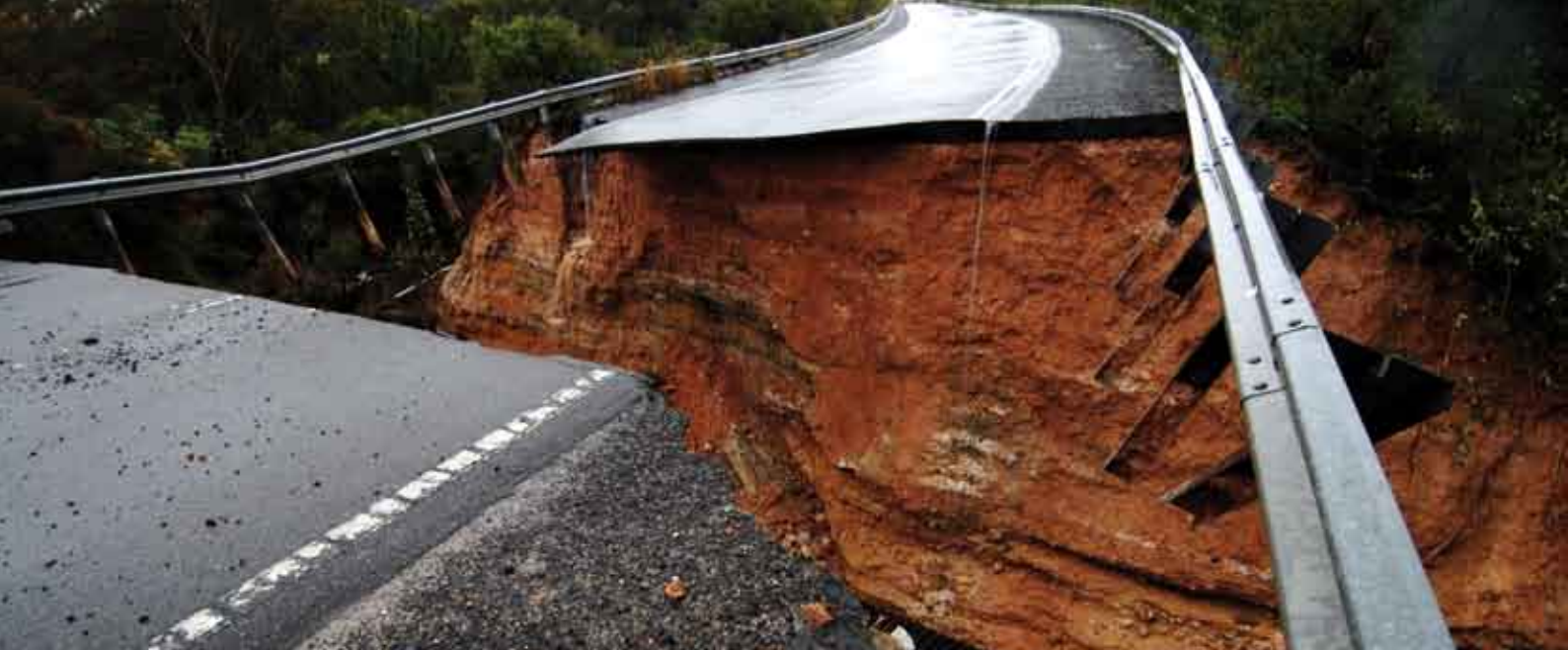
The collapsed part of the road along the Old Pacific Highway following a severe storm near Somersby in the central coast region, New South Wales, June 2007 Photo courtesy: AAP Image/Dean Lewins.
