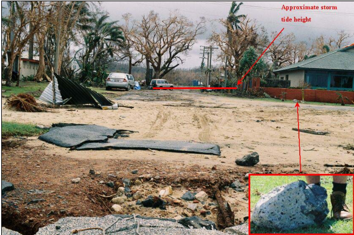
Coastal erosion and Storm Tide aftermath at Cowley Beach
