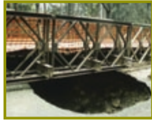
▲ Road collapse at Linea, Northern Tasmania, Australia. Copyright: Elerly Hamilton-Smith
