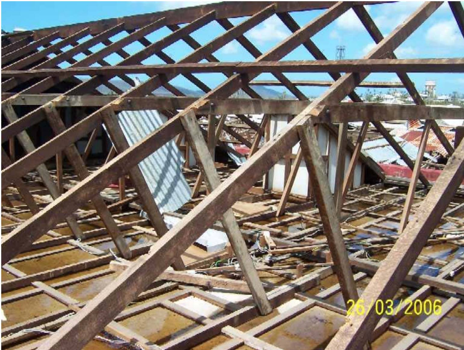
Roof damage to a residential house following Cyclone Larry, Innisfail. Image courtesy Geoscience Australia.
