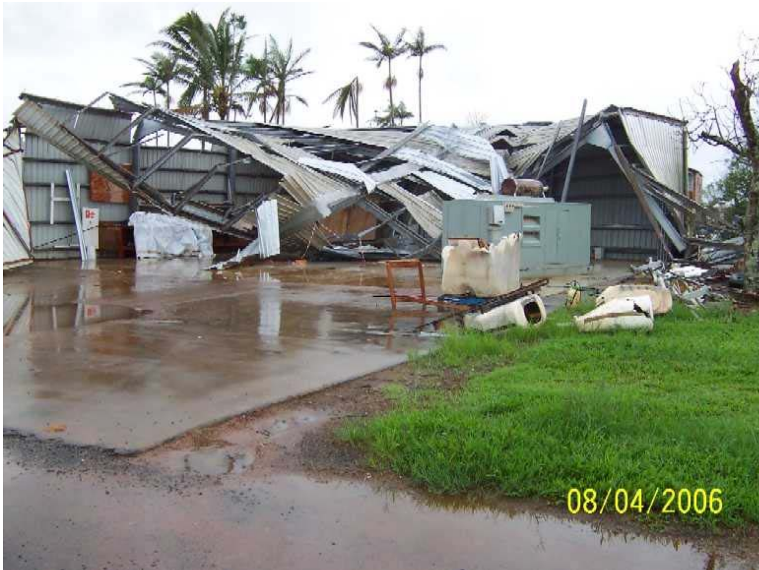
Destroyed industrial building following Cyclone Larry at an airfield near Innisfail. Image courtesy Geoscience Australia.
