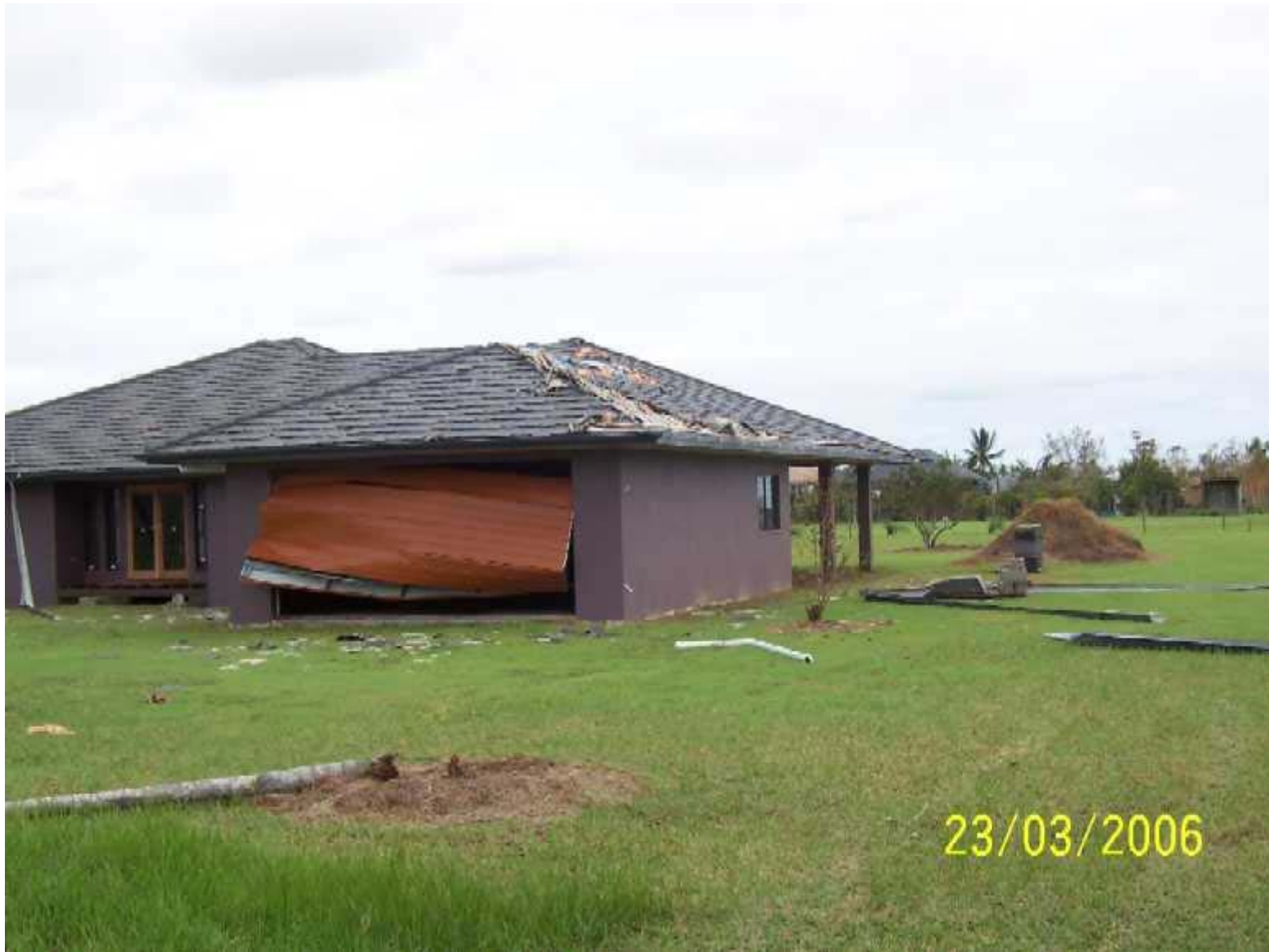
Damaged to a new residential building following Cyclone Larry, Innisfail. Image courtesy Geoscience Australia.
