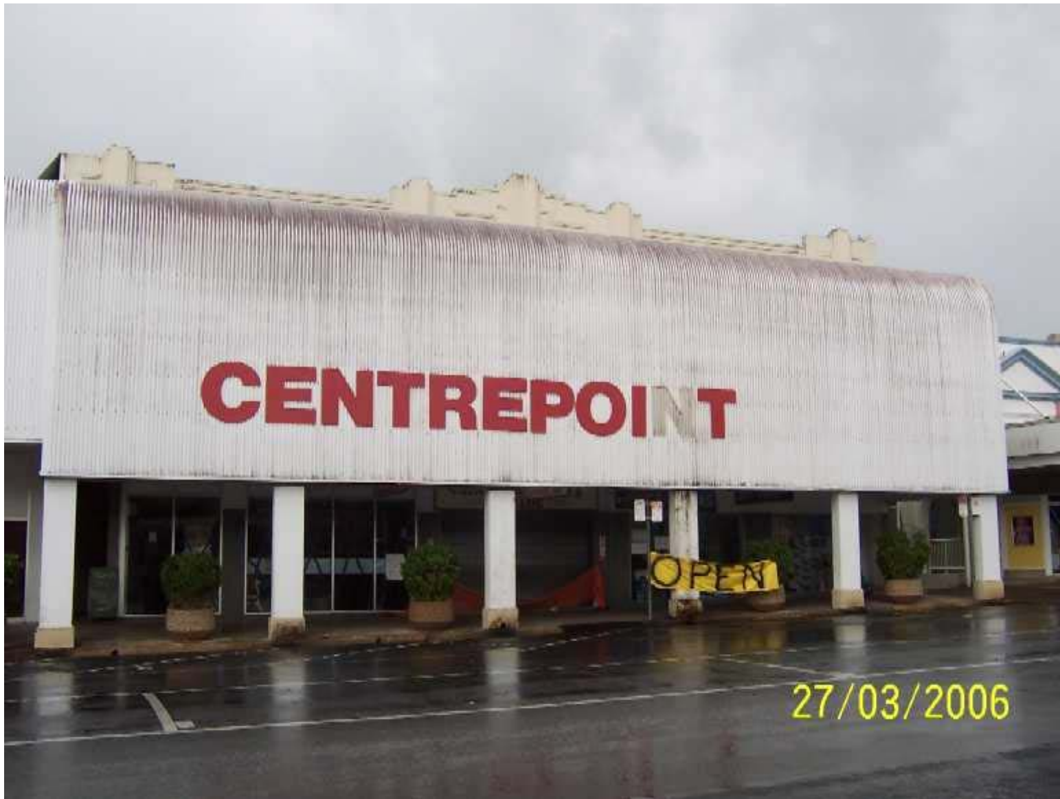
Commercial building damage following Cyclone Larry to "Centrepoint", Innisfail. Image courtesy Geoscience Australia.
