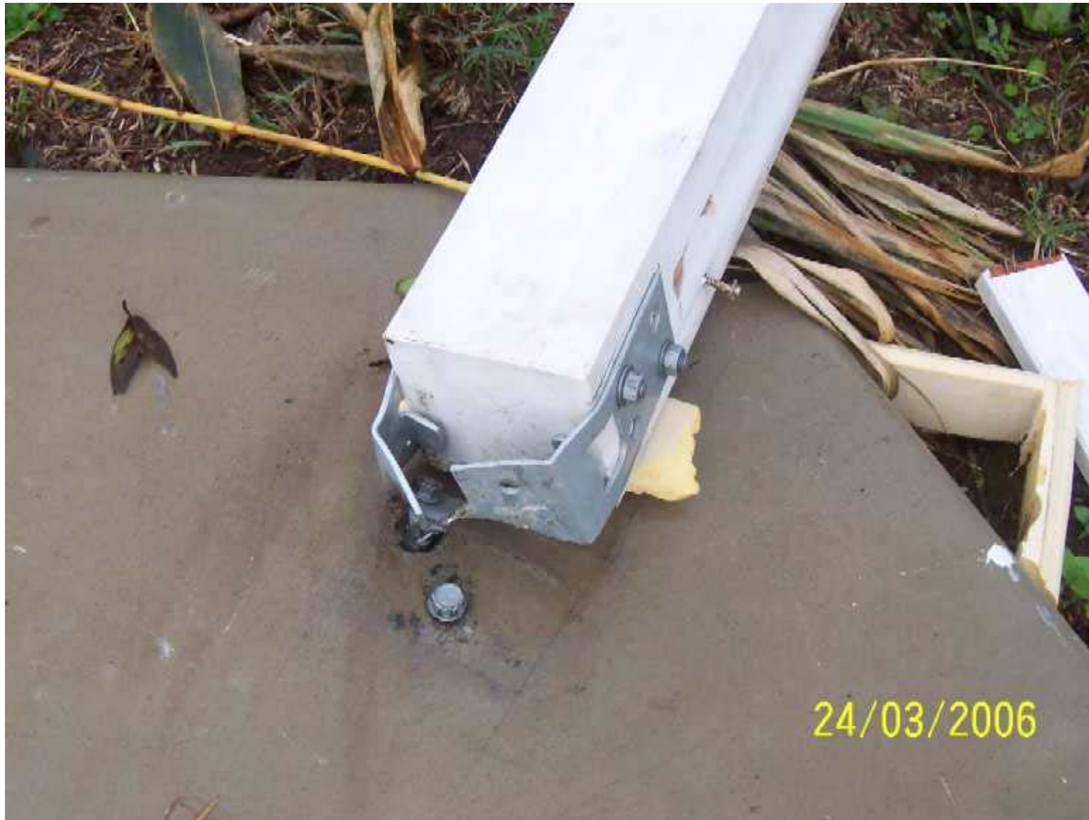
Damage to a veranda post following Cyclone Larry, Innisfail. Image courtesy Geoscience Australia.
