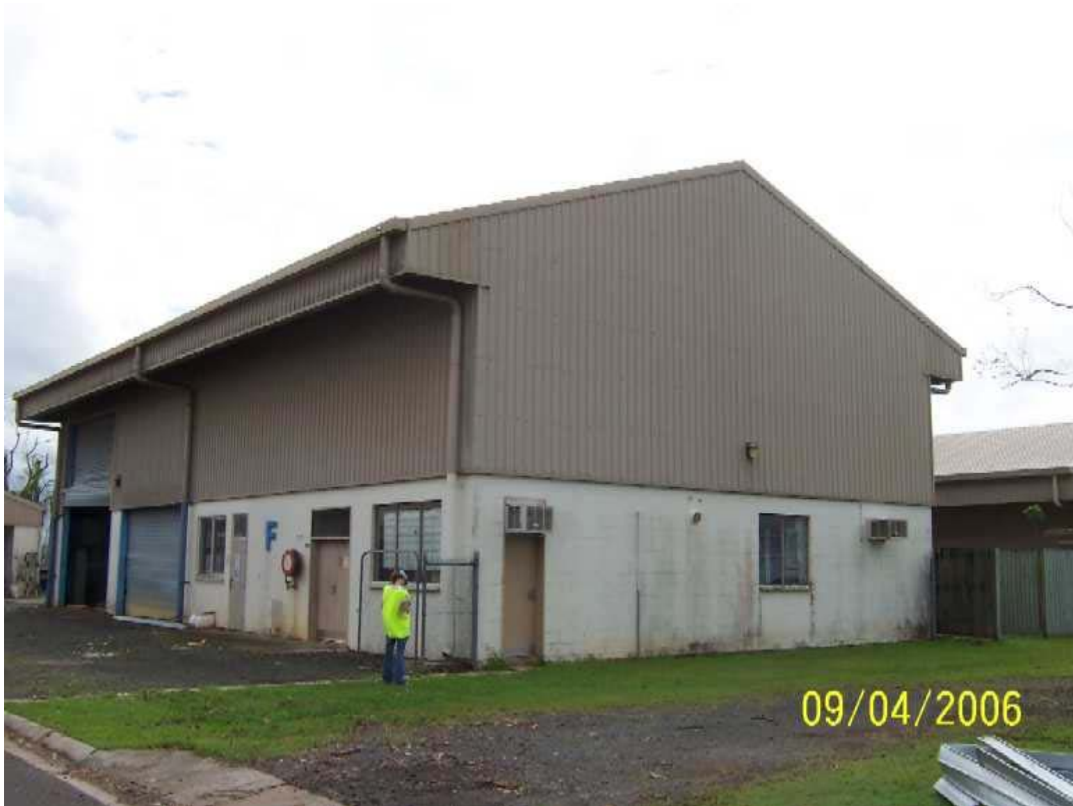
GA team member surveying damage to an industrial building following Cyclone Larry, Innisfail. Image courtesy Geoscience Australia.
