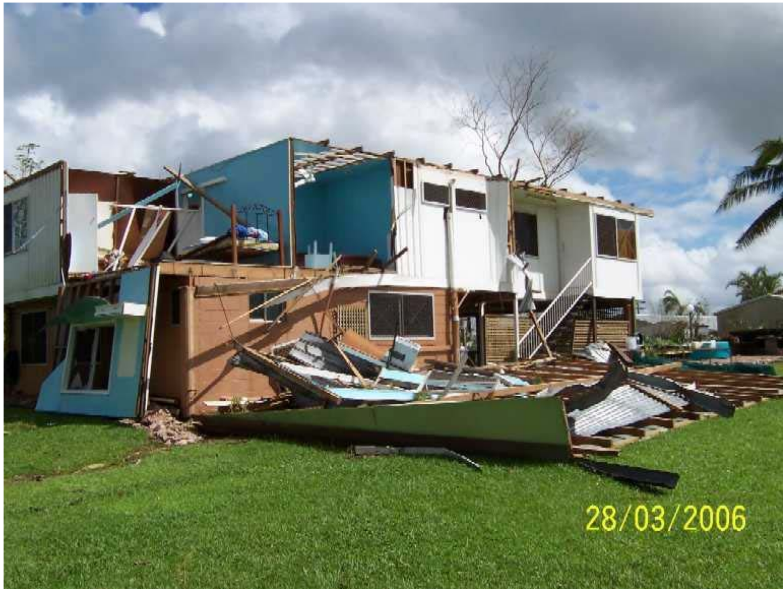
Severely damaged residential building following Cyclone Larry, Innisfail. Image courtesy Geoscience Australia.
