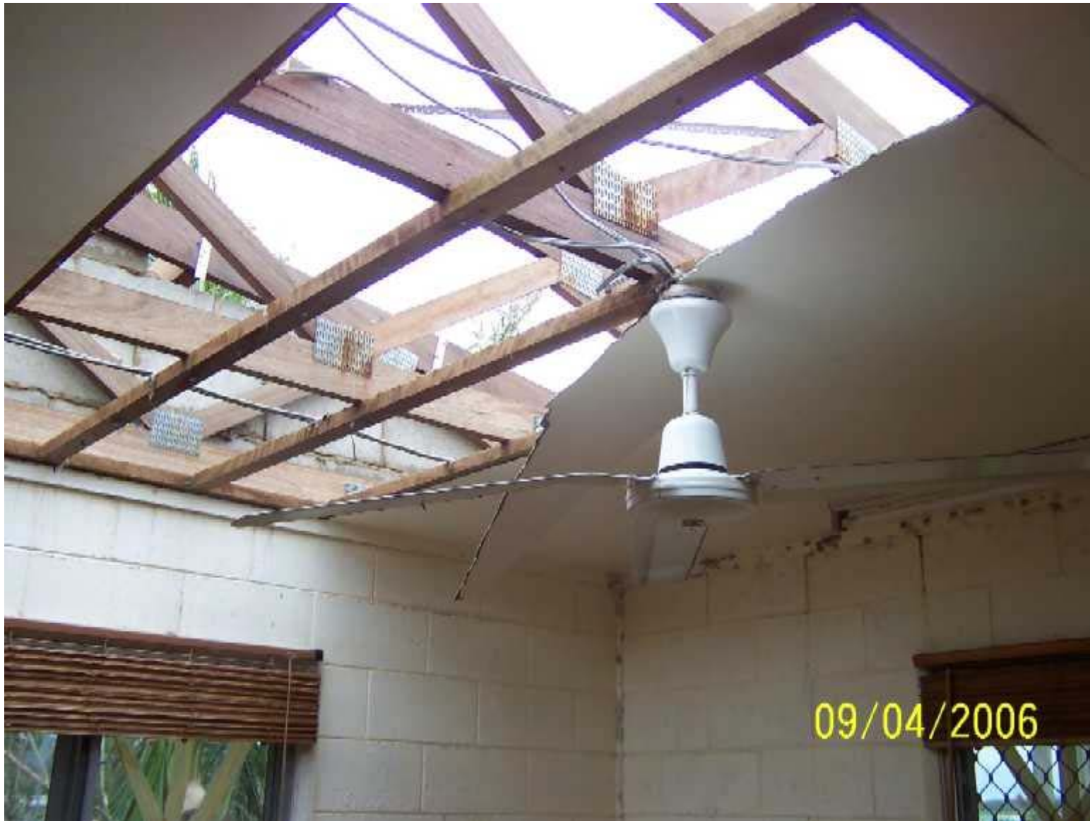
Internal damage to a residential house following Cyclone Larry, Innisfail. Image courtesy Geoscience Australia.
