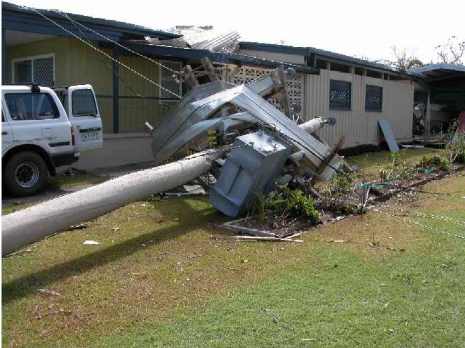
Power pole damage to a residential building following Cyclone Larry, Innisfail. Image courtesy Geoscience Australia.
