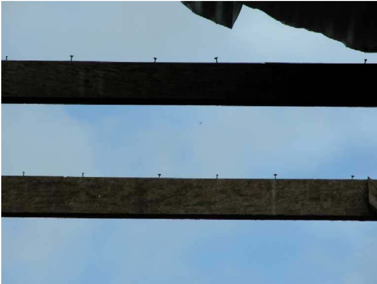
Flimsy nails used in the construction of a residential house, Innisfail. Image courtesy Geoscience Australia.
