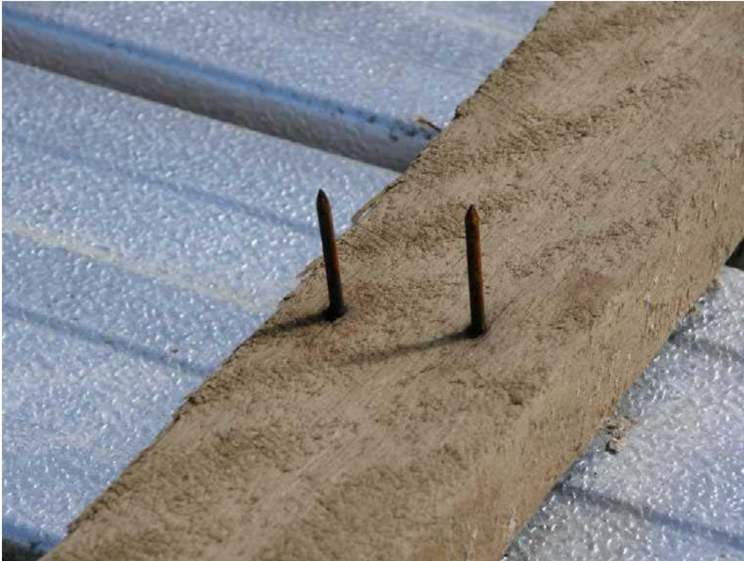
Rusted nails used in the construction of a residential house, Innisfail. Image courtesy Geoscience Australia.
