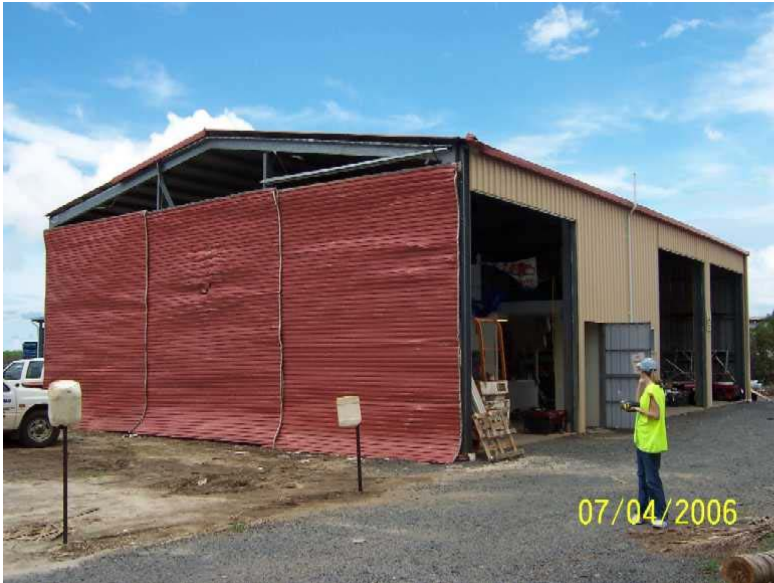
Industrial building damage to roller doors following Cyclone Larry, Innisfail. Image courtesy Geoscience Australia.
