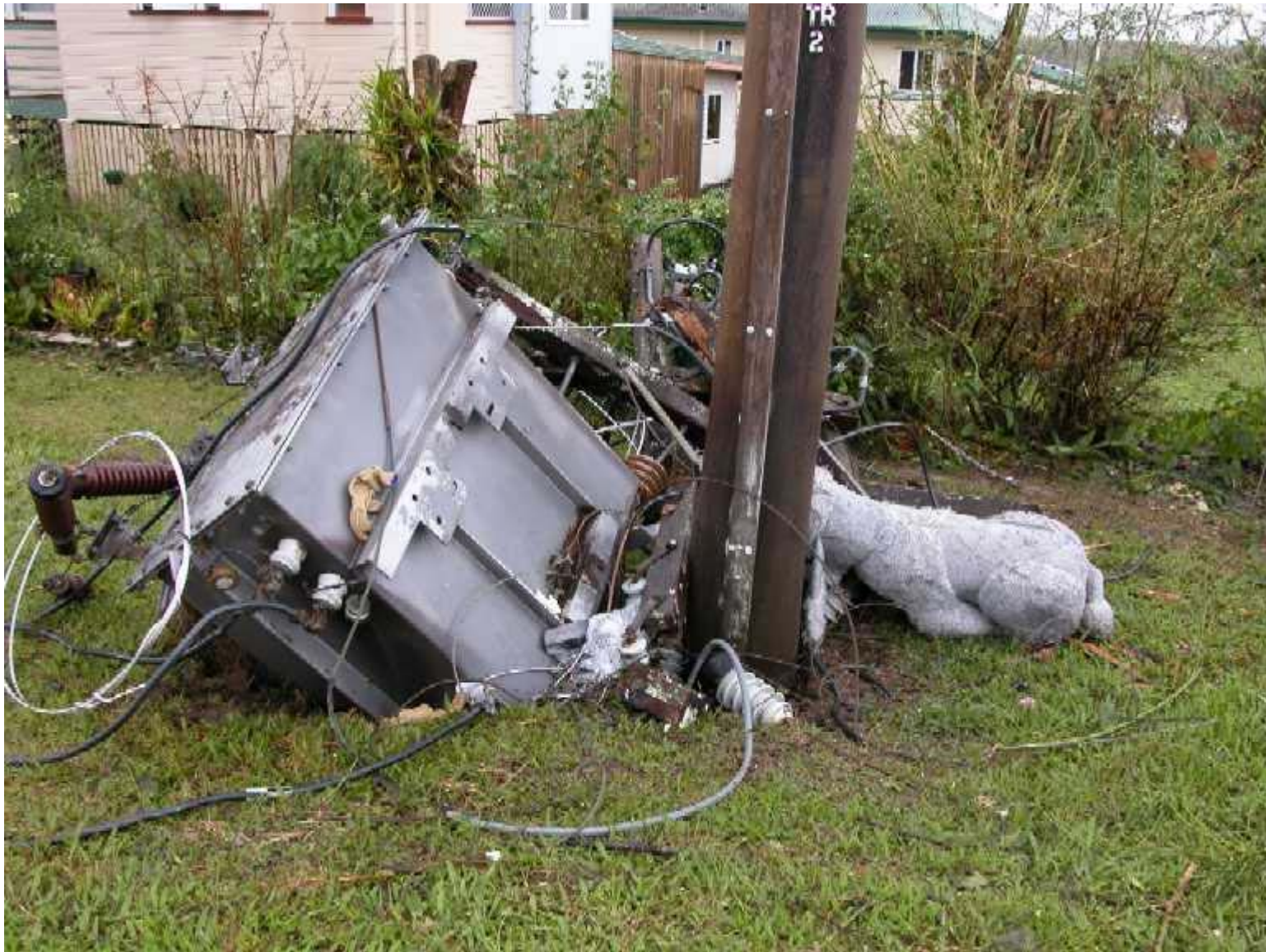
Damage to power supply in Innisfail following Cyclone Larry. Image courtesy Geoscience Australia.
