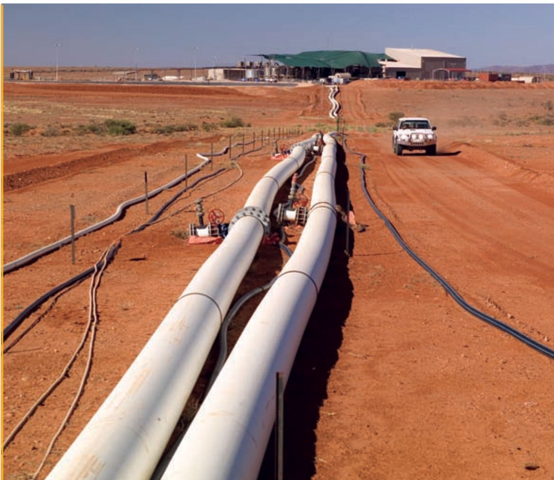
Trunk lines and processing plant at Beverley in situ recovery uranium mine, South Australia (Heathgate Resources Ltd).
