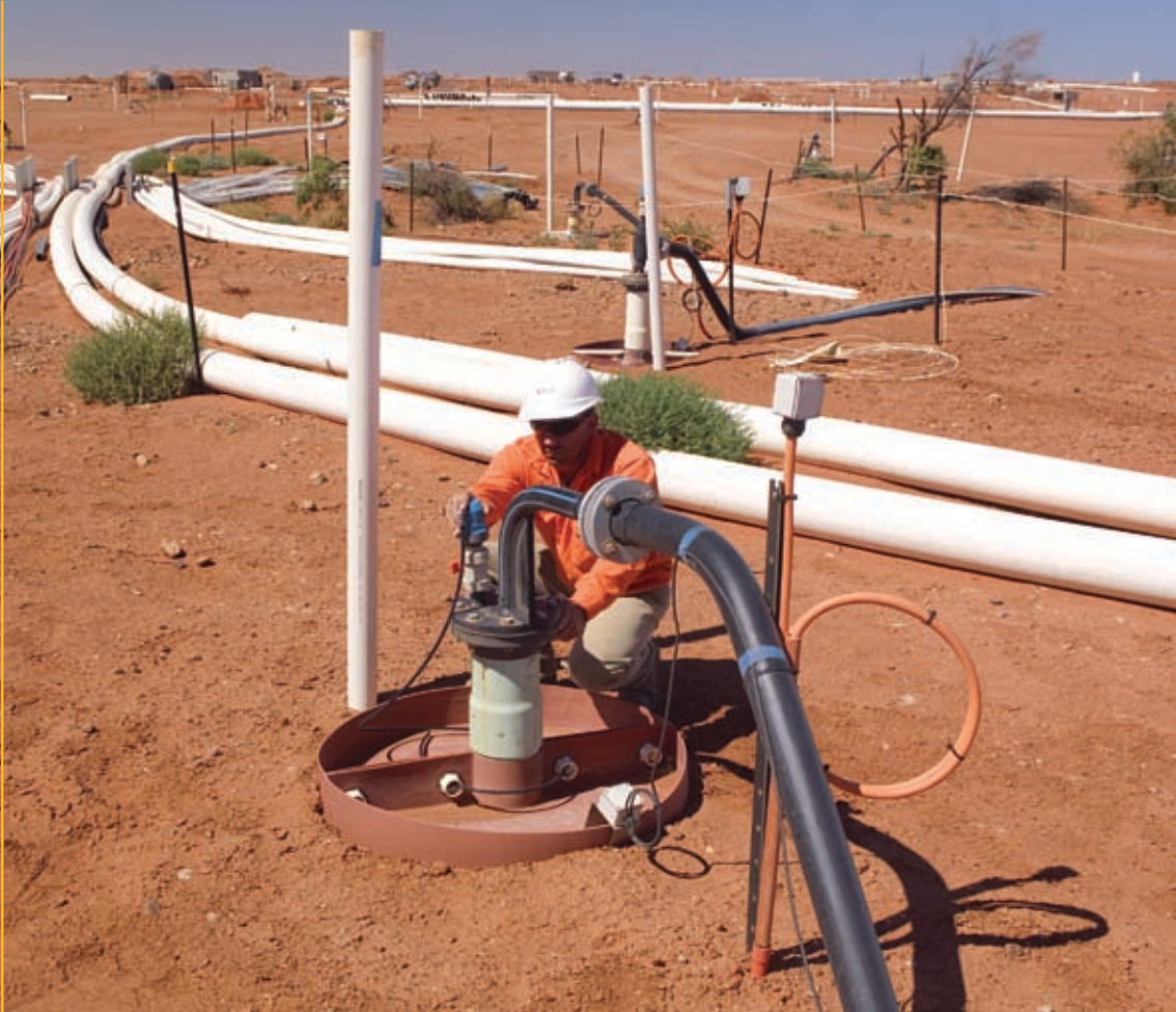
Wellfield and injection well at Beverley uranium mine, South Australia (Heathgate Resources Ltd).
