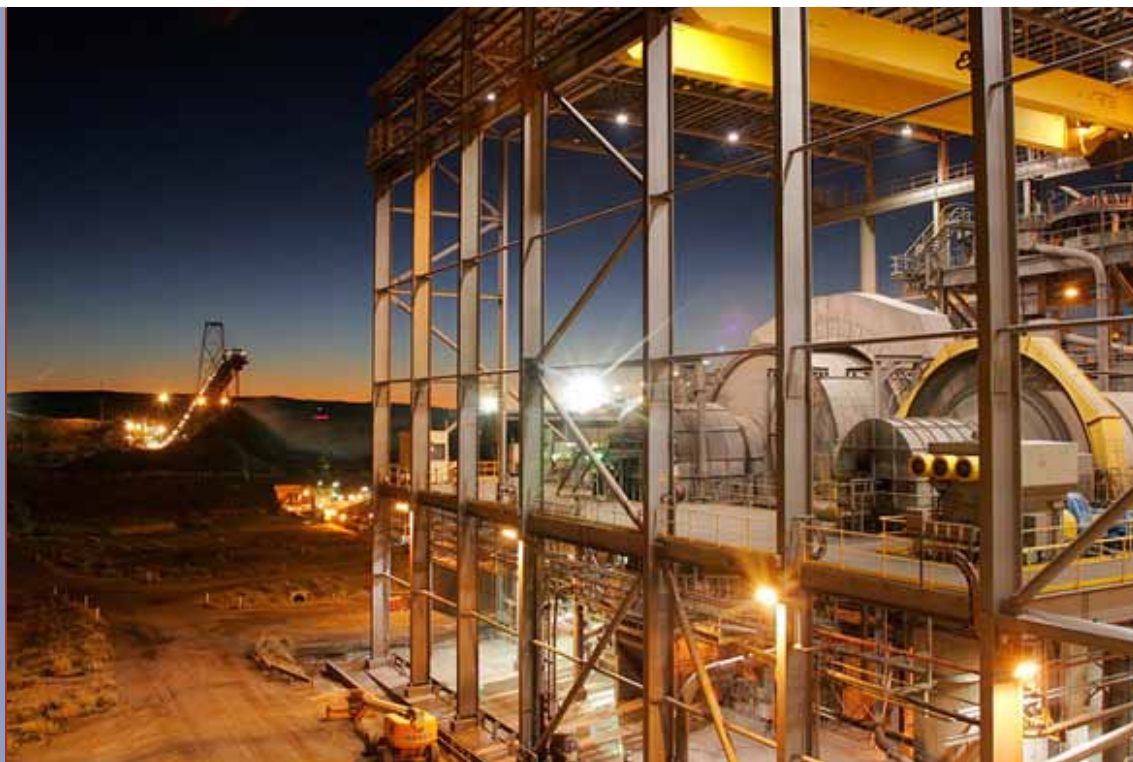
Semi-autogenous grinding mills at metallurgical processing plant, Century zinc-lead mine, north Queensland (Minerals and Metals Group Ltd)
