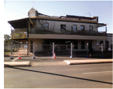
Figure 2. Damage caused to a hotel in Boulder. The damage is typical for two storey unreinforced masonry buildings with toppling of parapets either outwards into the street or inwards through the roof. This building also sustained other types of damage such as cracking over doors and windows and substantial cracking to internal masonry walls.
